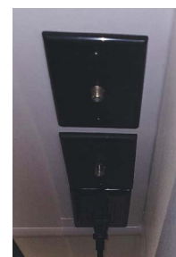
ANTENNA POWER SUPPLY
