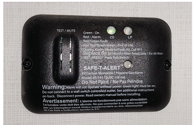
THE CO AND PROPANE GAS ALARM. SEE SECTION 46 FOR ITS LOCATION IN THE RV.
