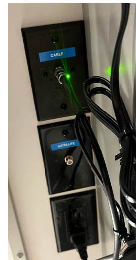
ANTENNA POWER SUPPLY
