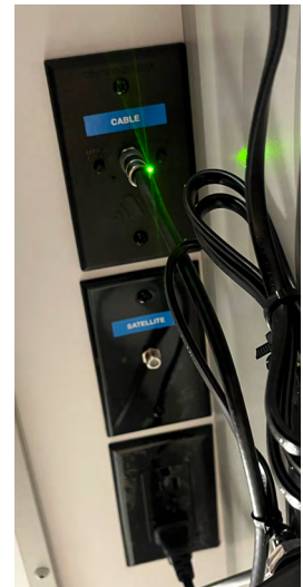
ANTENNA POWER SUPPLY
