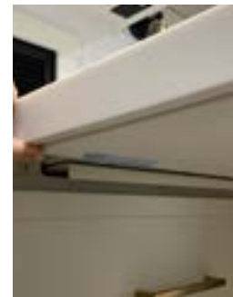
NOT LOCKED IN PLACE
