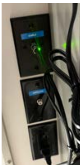
ANTENNA POWER SUPPLY
