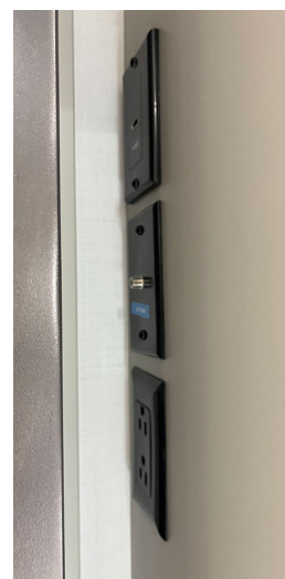
ANTENNA POWER SUPPLY
