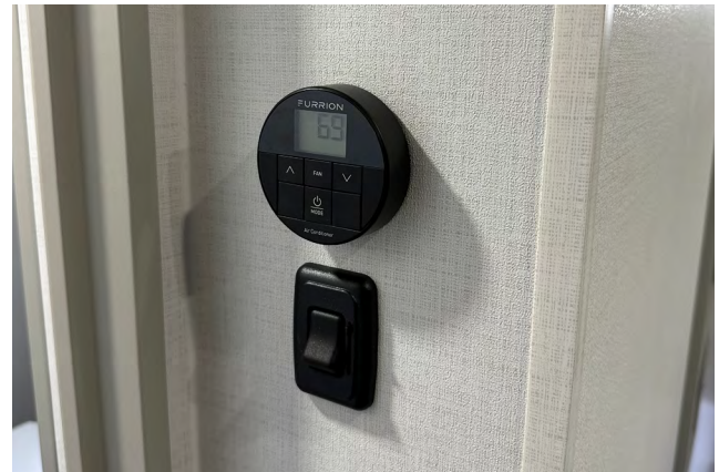
The bedroom thermostat is located just inside the bedroom door on the bathroom wall.
