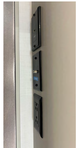
ANTENNA POWER SUPPLY
