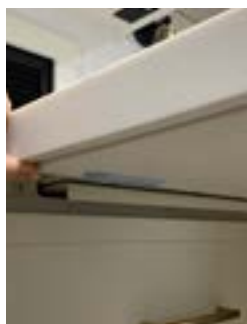
NOT LOCKED IN PLACE
